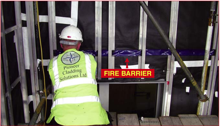
EXTERNAL FIRE BARRIER FITTED TO ESCAPE ROUTES
