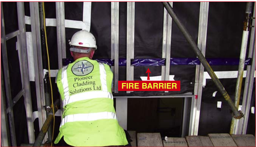
EXTERNAL FIRE BARRIER FITTED TO ESCAPE ROUTES
